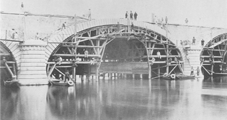
Hippolyte Collard, Removal of the Centering—View of Arch No. 4 Taken from Downstream, 1865 , from Pont de Bercy , 1865, pl. 5.
